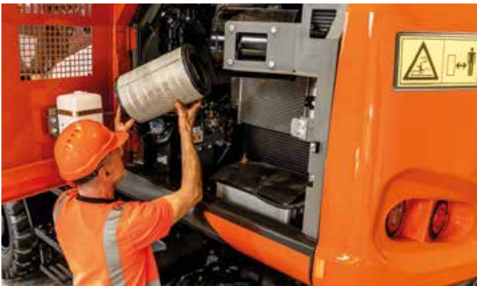
Maintenance is easy at ground level.
